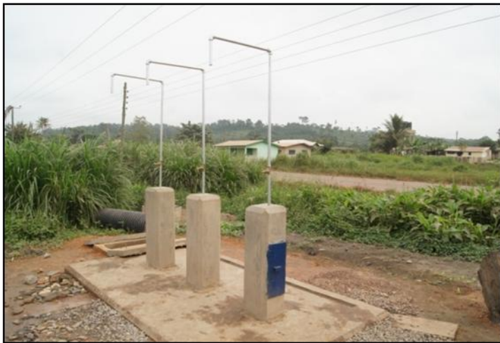
Plate 3: Small Town Water Supply System
