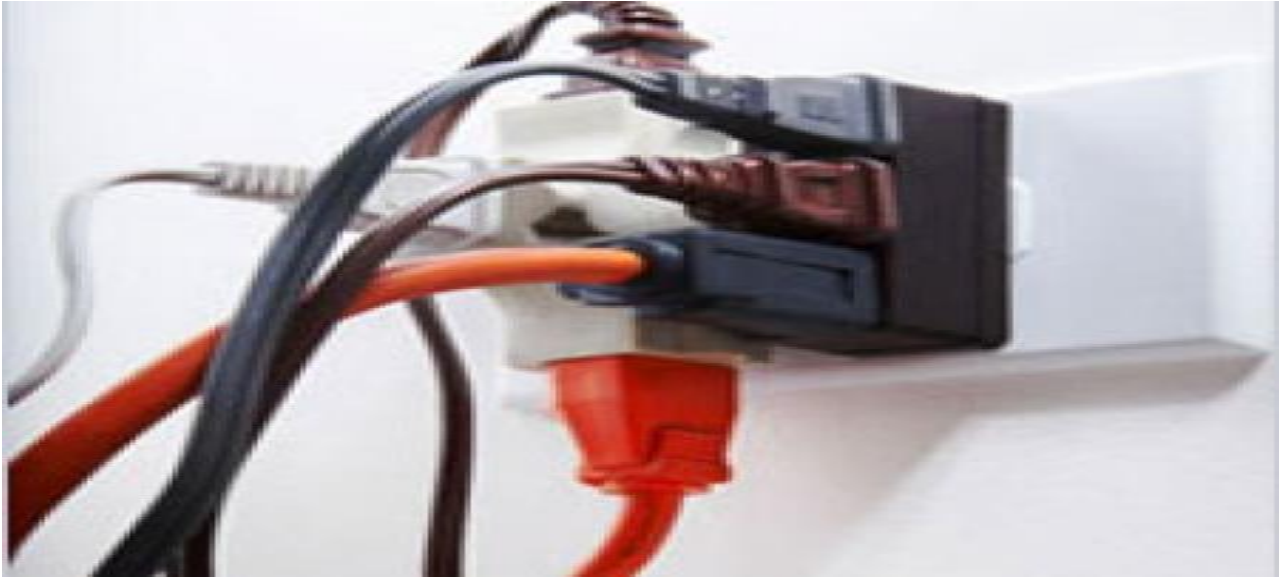
Plate2: a photograph having multiple plugs in a socket
