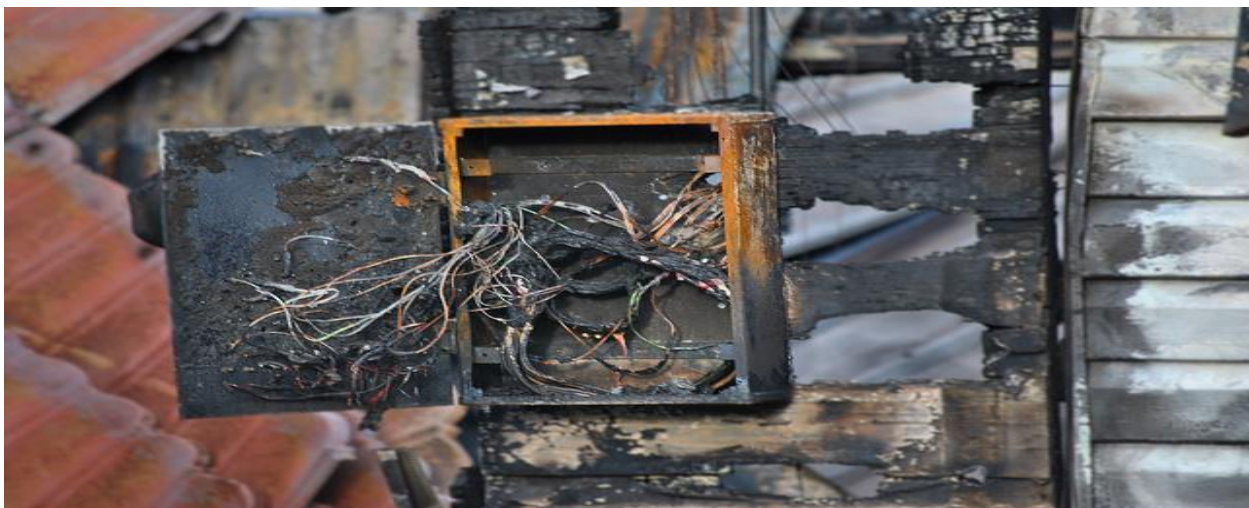
Plate2: A photograph showing burnt electrical outlet
